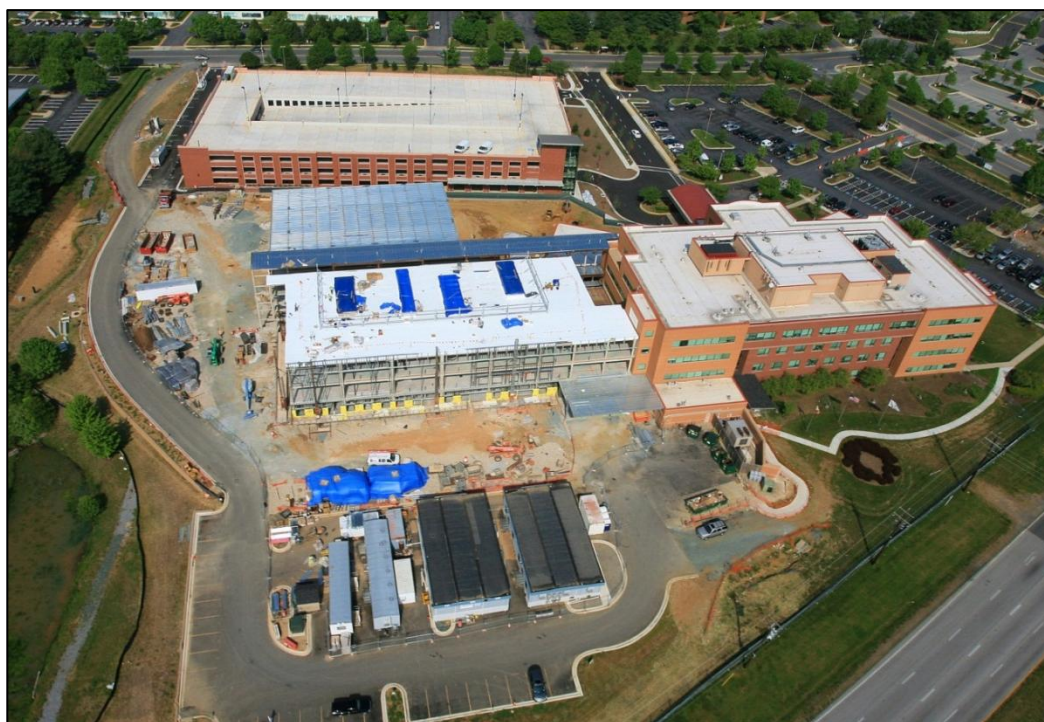
Figure 7 - An aerial progress photo taken on April 21, 2012 shows the temporary roof just 12 days after its construction began. Take notice that there is no framing on the east façade. Image courtesy of DPR Construction.
