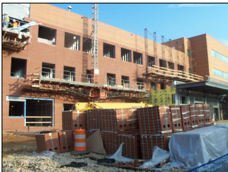
Figure 3 - The east elevation is shown almost completed. A Fraco lift can be seen in the center, with a Mason King manual cranked scaffold equipment sits on the canopy roof. Notice the amount of space currently taken up by the mason subcontractor. Personal photograph taken by Chris Pozza.
