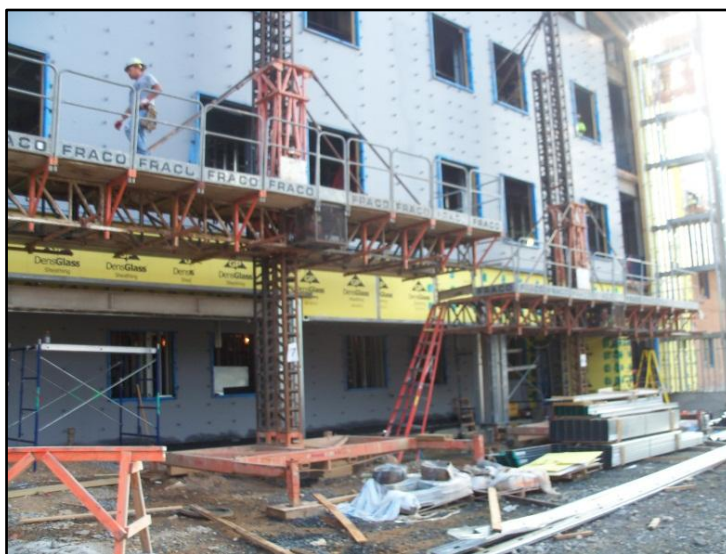
Figure 4 - Image taken the same day as Figure 10. Masons preparing for the next phase at the south elevation. Work can never take place underneath Fraco Lifts. Personal photograph taken by Chris Pozza.
